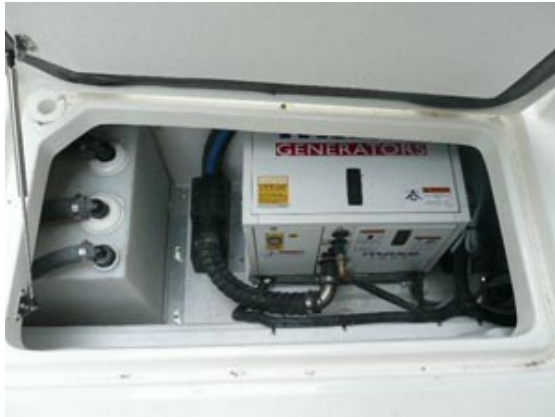
Mase Generator Control Panel under AC/DC Panels
